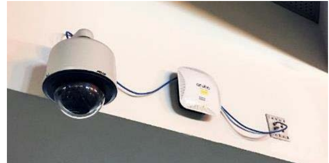
Photo taken at McCarran Airport in Las Vegas by our awesome marketing person – Anyone could jump up and pull out the patch cord to the surveillance camera and wireless access point.
