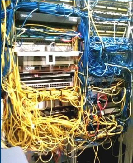
Poor cable management
