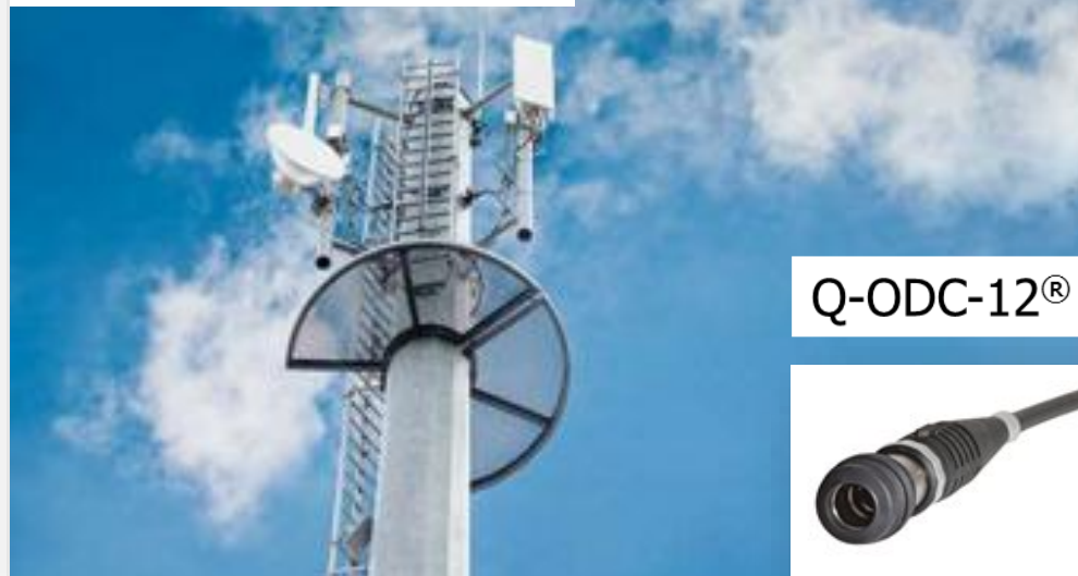
Fiber to the Antenna (FTTA)
