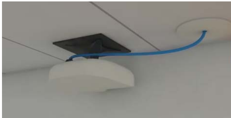
Direct Connect Horizontal Cabling to WAP
